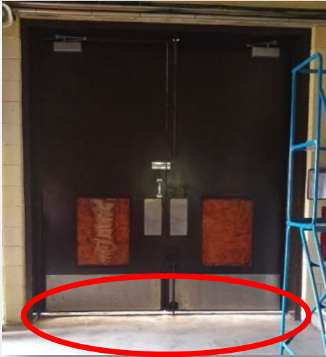
Fix gaps around doors.
