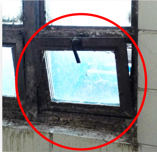
Hard to reach windows in outbuildings are opened in the summer and then left open in the winter. Stack effect can increase heat losses.
