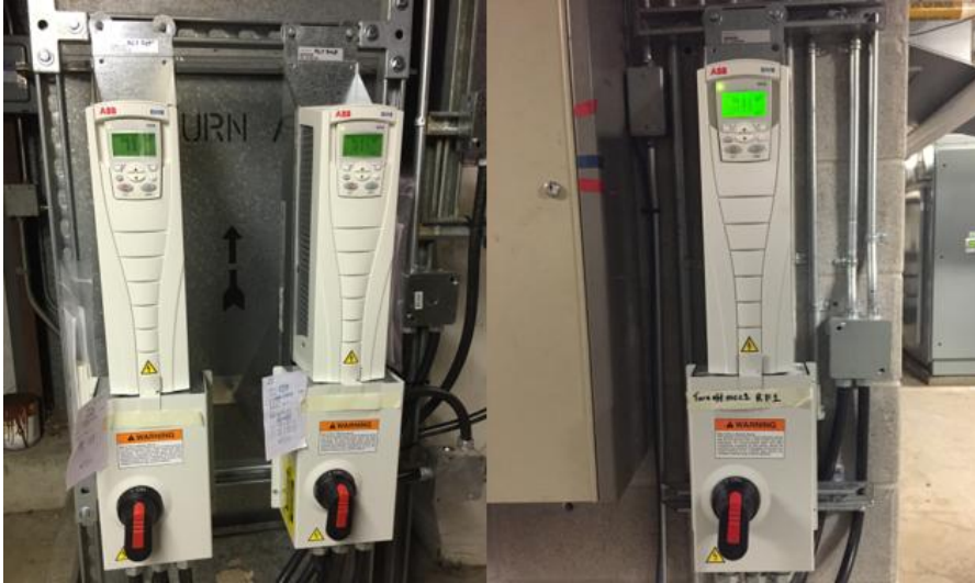
VFD units on AHUs at Ajax & McLean Community Centres
