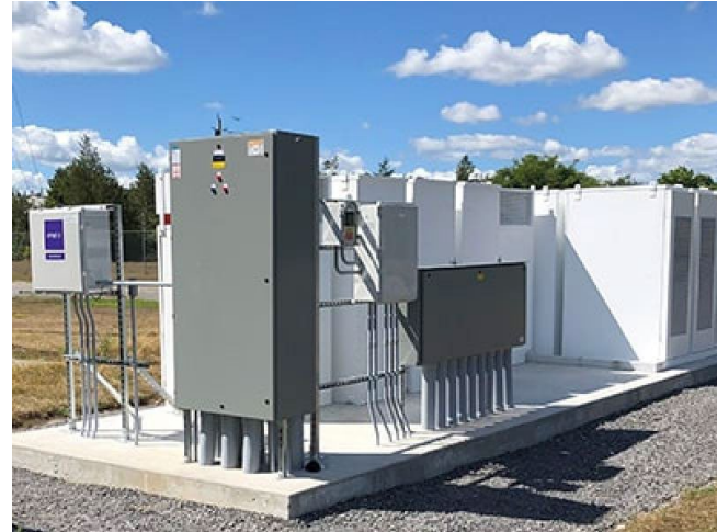
A battery storage system for Berry Global in Belleville, Ont. (Courtesy Enel)
