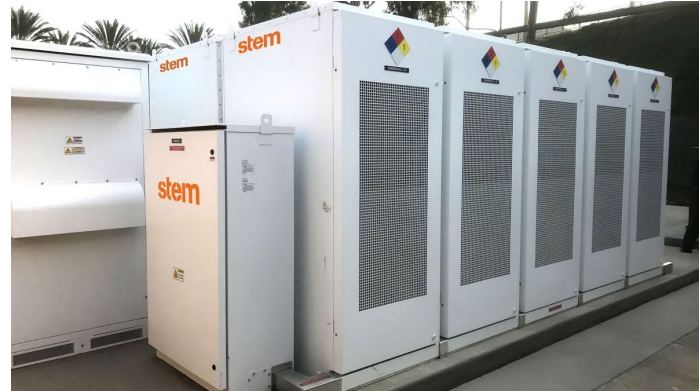
A STEM battery storage system (Courtesy Utility Dive)
