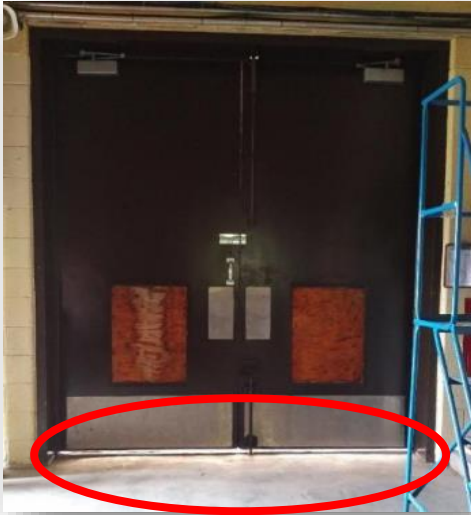
Fix gaps around doors.
