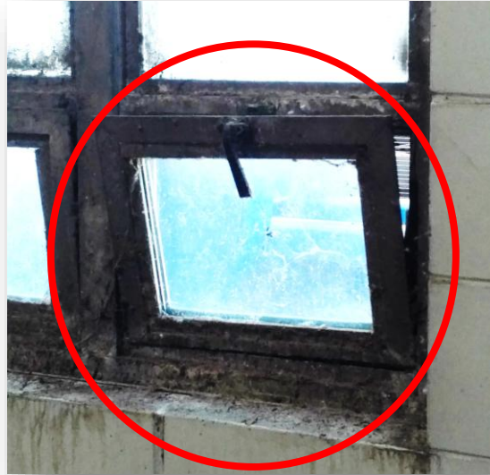
Hard to reach windows in outbuildings are opened in the summer and then left open in the winter. Stack effect can increase heat losses.
